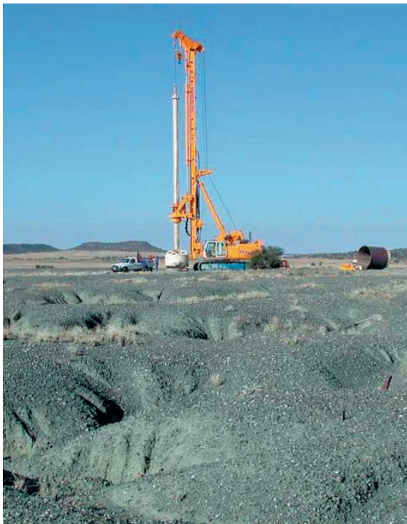
Bulk sampling of mine dumps is an ideal application for the BG 36 kelly drilling rig 2,5 m diameter sample holes in Kimberly, South Africa
