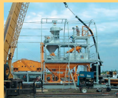
Desanding plant and kimberlite recovery system BEK 375
