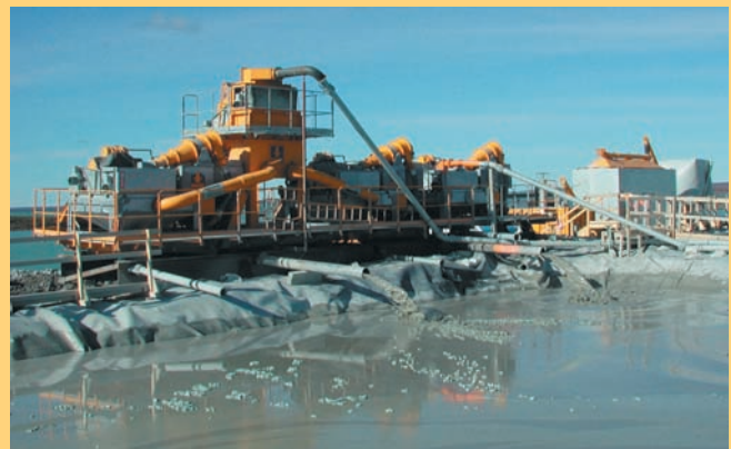
Slurry desanding plant BE 500 (capacity 500 m 3 /h) at DIAVIK, Canada
